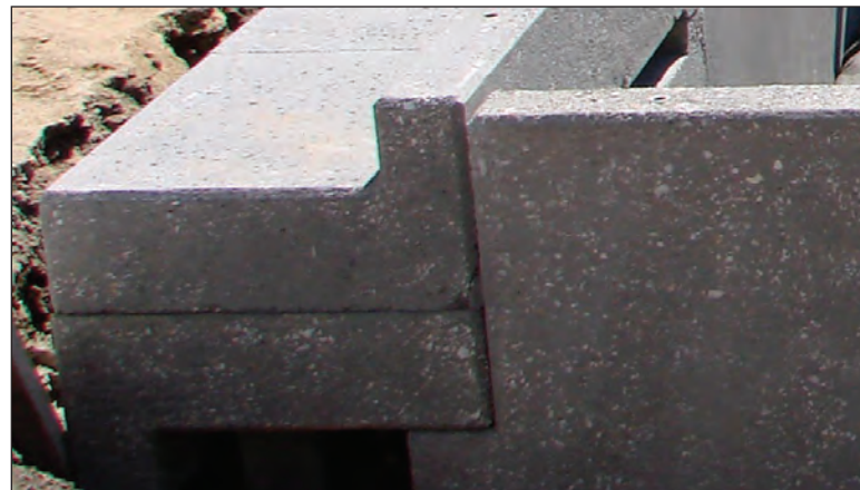
Step 8: Install the water intake structures using the N• Modules as shown in Stage 3-D.
