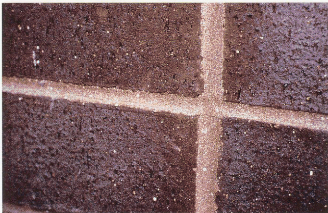
Fig. 4. The use of a strong acid cleaning solution has etched the surface of these mortar joints, exposed sand particles, and significantly changed the appearance of the mortar joint.
