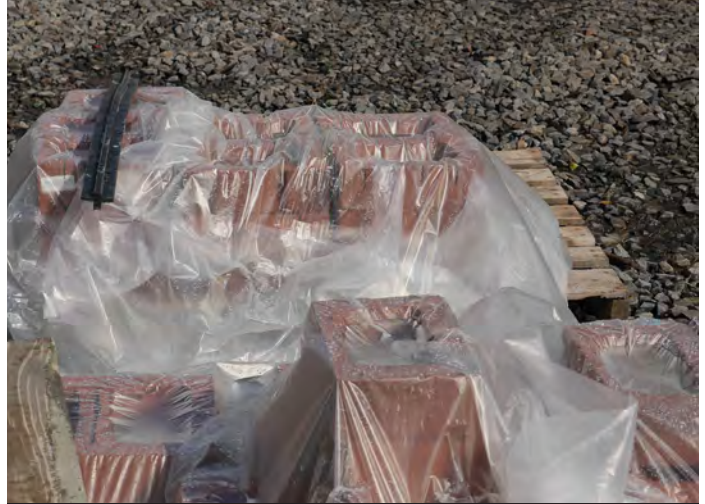
Materials should be stored on pallets and protected from the elements while stored on site
