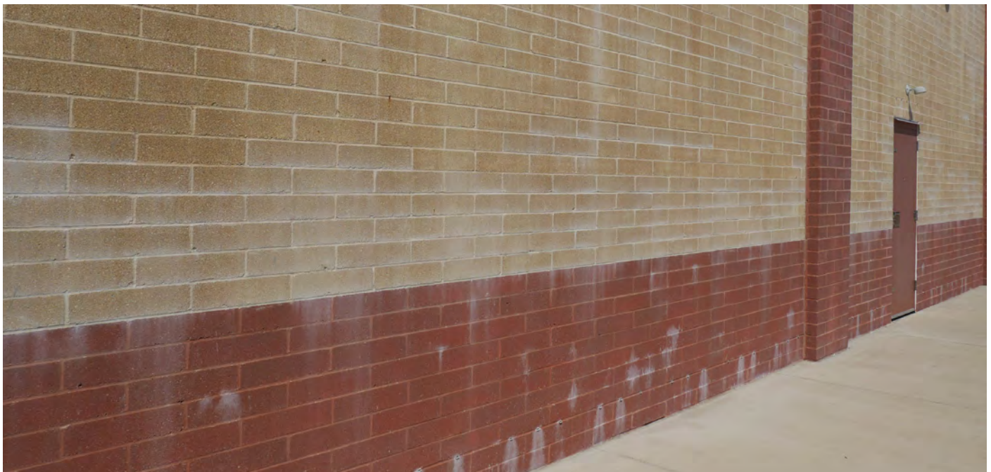
A failure to protect the exposed wall tops from rain during construction can lead to the wall's empty cores filling with water, which as it drains out of the wall leaches salts from the concrete which results in efflorescence forming on the exterior. This makes cleaning the wall much more difficult
