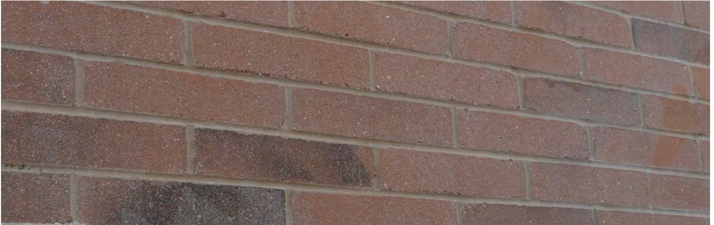
Cleaned Wall Section showing discoloration and damage due to use of high pressure rinse - note the wand marks where the wall was particularly hard hit (water pressure was 500 psi)
