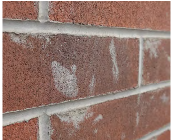
Mortar Stains Prior to Cleaning
