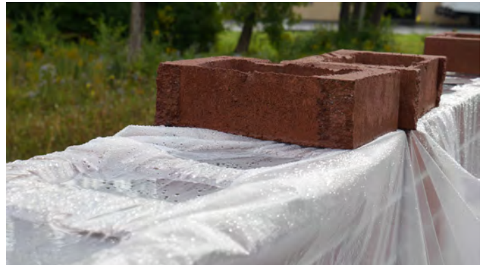
Wall top tarped to protect against rain during a break in construction.
