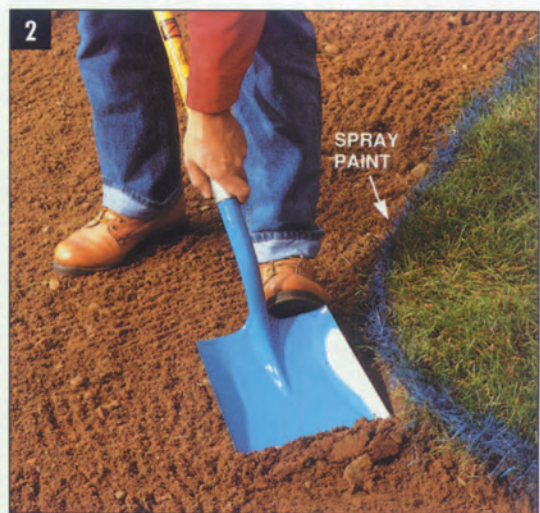
2 REMOVE SOD in an area extending 8 in. beyond the boundaries of the patio. SPRAY PAINT indicates the excavation line.
