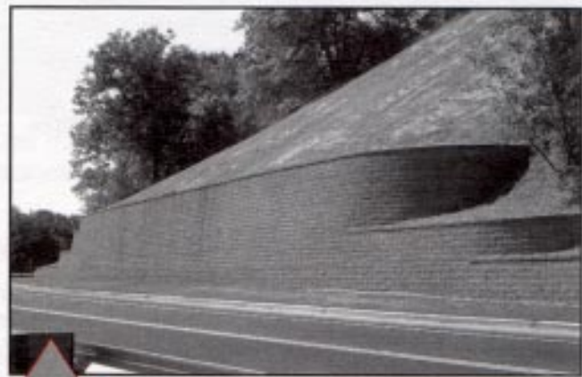
Return walls create a terraced appearance instead of a series of short steps at the top of the wall.
